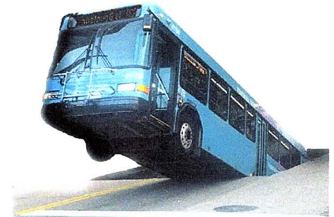
The pothole that ate a Pittsburgh Bus!
